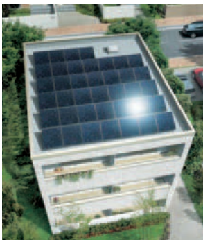
Fixed-installation solar panels
