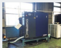
Ironworks compressor (replacing equipment with high-efficiency models)
