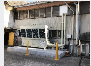
The new chiller
