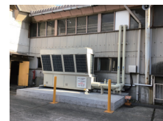
The new chiller
