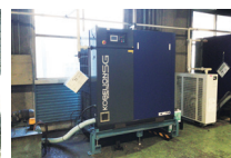
New compressor in the ironworking plant
