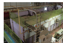
Exterior-clad insulation on the drying furnace door
