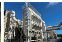
Woodworking dust collector (replacing equipment with high-efficiency models)
